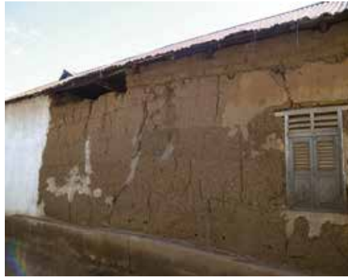
A building damaged by blasting
